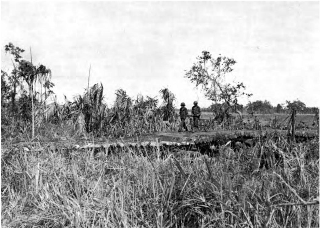
BRIDGE OVER SIMEMI CREEK. New Strip in the background. (Photograph taken after bridge was repaired by the 114th Engineers.)
